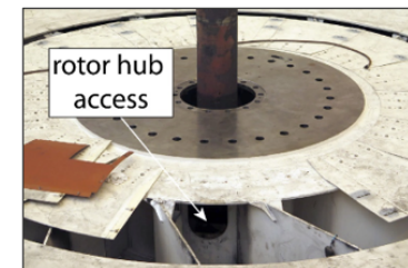
Figure 1- Rotor hub access panel removed
