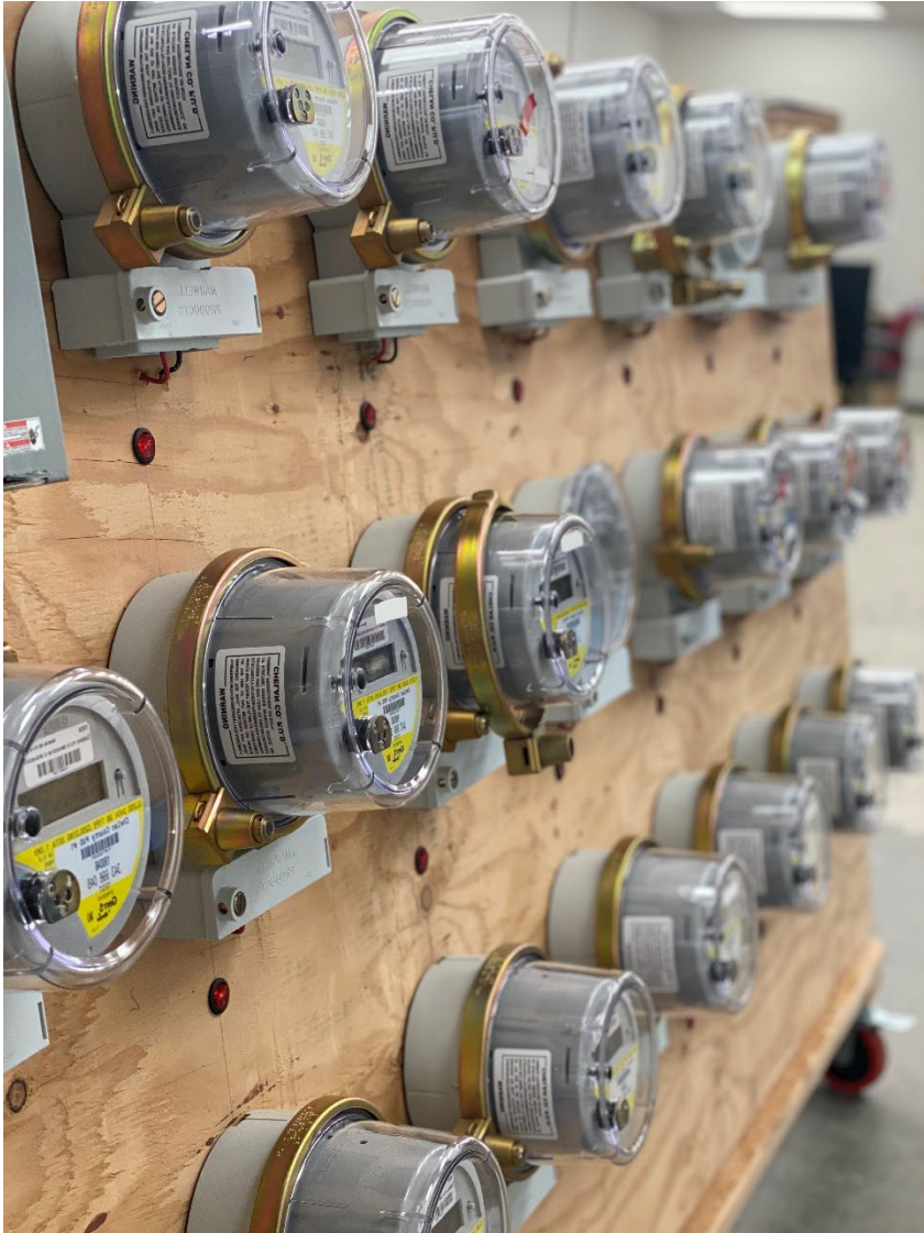
New Itron AMI meters – under testing
