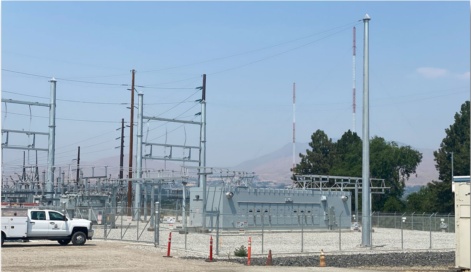
Photo: Hawley Substation
