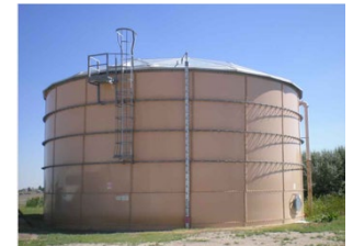
Above-ground storage tank
