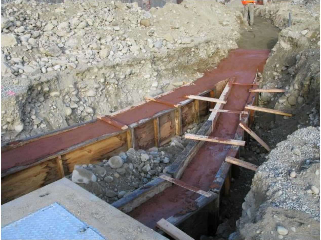
Conduit road crossings, formed up and red-dyed concrete placed. Picture taken on 12/11/08.
