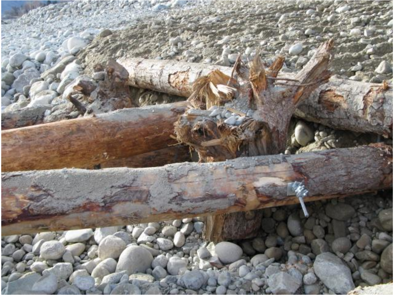
This picture is of a completed V-Log Jam in the habitat channel. Picture was taken on 12/2/08.
