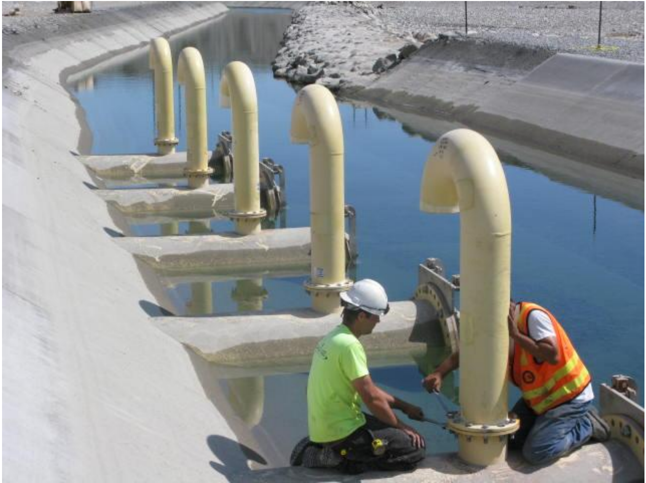
The air relief pipes are being installed on the 42" diameter discharge pipes at the pump station. Picture was taken on July 9 th , 2009.
