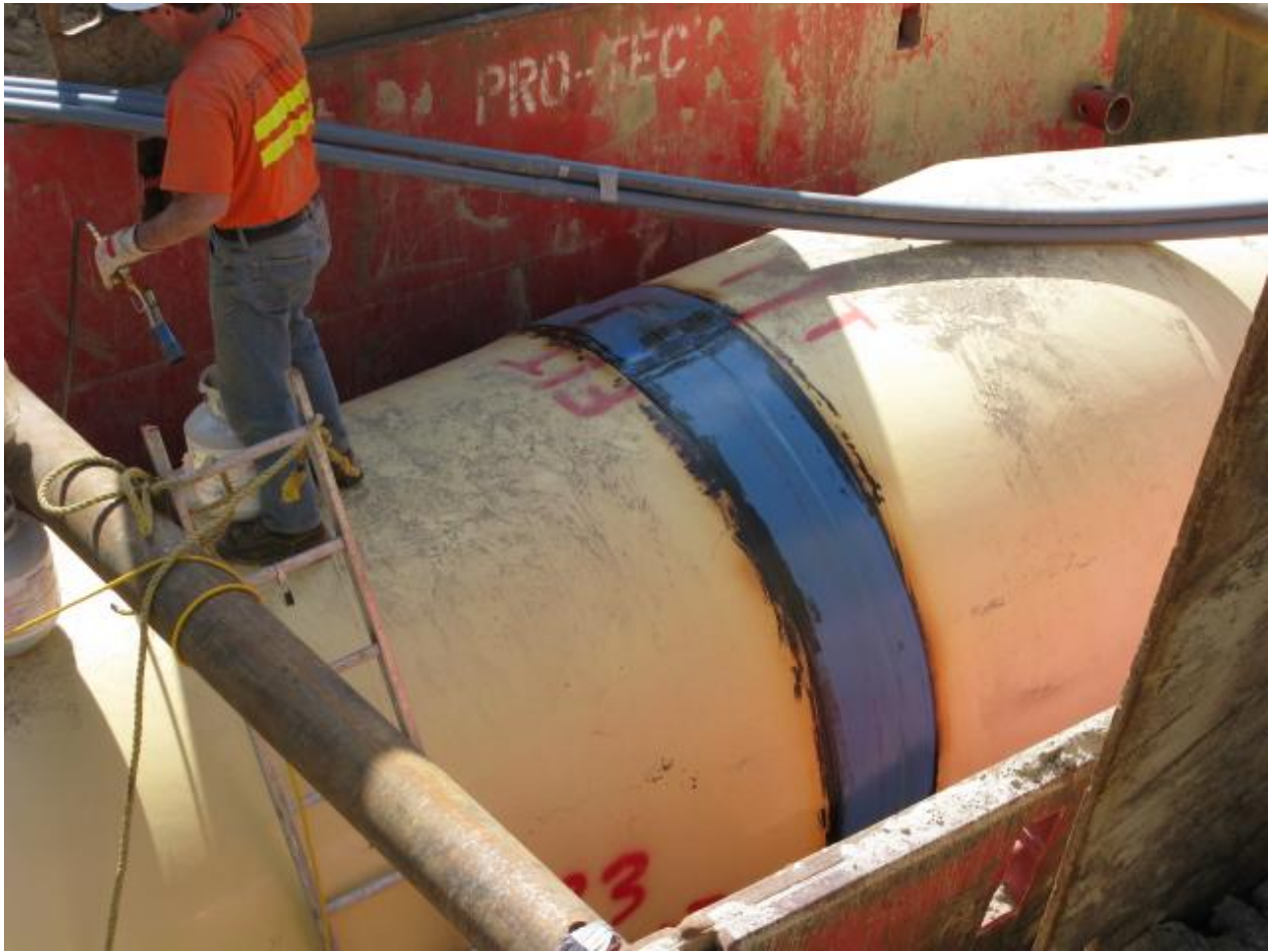
This picture shows the 85" diameter LLO piping. A completed heat-shrink sleeve has been installed over a welded joint. Picture taken on 4/16/09.
