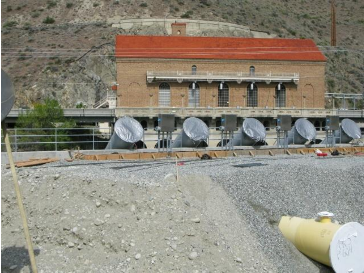
Picture taken on 5/7/09. This photo shows one of the backfilled 42" diameter discharge pipes (yellow piping). Forms are installed for the sidewalk along the retaining wall. Notice the pump tubes are covered, awaiting installation of the pumps.
