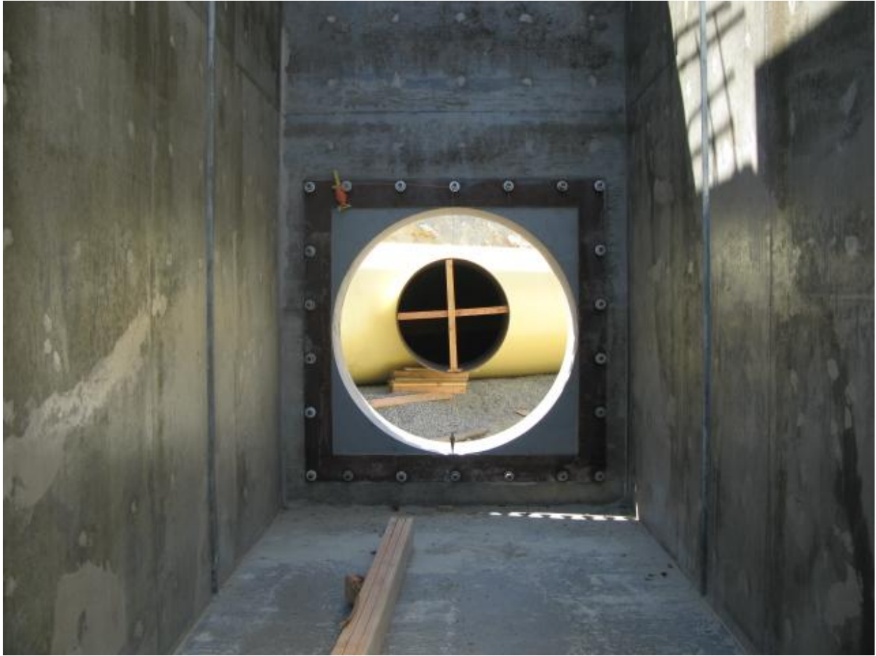
This is looking upstream through the low level outlet (LLO) outlet structure. View is through the concrete penetration for the valves, to the outlet piping. April 24, 2009.
