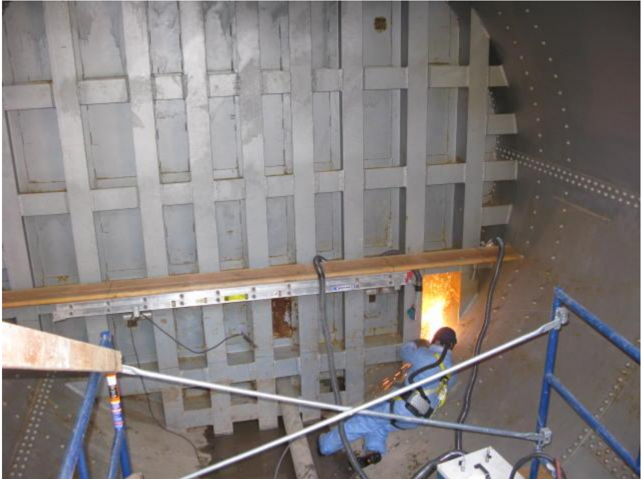
This picture was taken on 3/10/09. After the sheet pile wall was cut open, work removing the beams from the bulkhead steel began.
