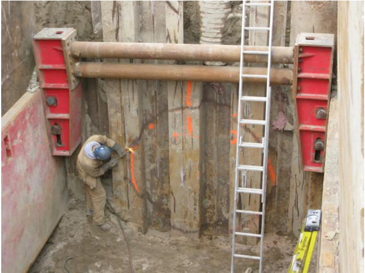
This is a picture from 3/9/09, of the sheet pile wall, with the dry tunnel and bulkhead for the 17-foot diameter penstock behind. The hole being cut is for the eventual LLO pipe installation.
