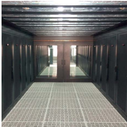
Datacenter Cold Aisle Internal
