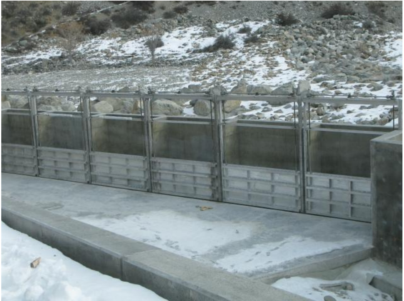
This is a photo of the aluminum slide gates at the Canal Outlet Structure. Picture was taken on 1/29/09. The walkway and gate operators have not yet been installed.
