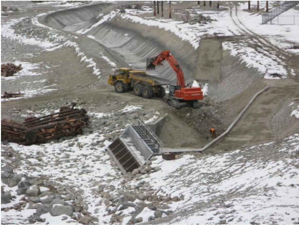
This shows Reach 4 looking south, on February 10 th , 2009. Notice that the slide gates have been installed. Also, excavation work is underway towards completing the conveyance canal tie-in to the outlet structure.
