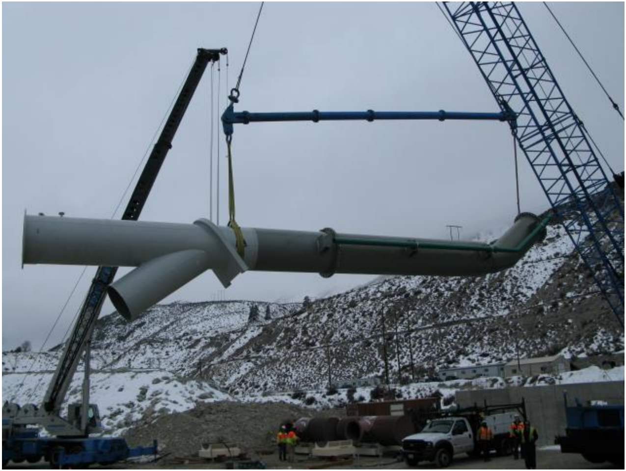
This picture shows the setting of the first pump tube, on 1/21/09. Notice the 6" air burst piping mounted to the side of the pump tube.
