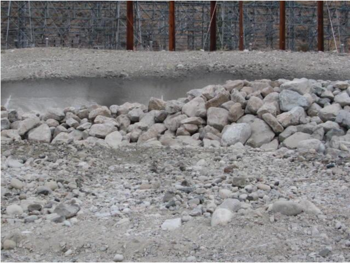
Rip-rap slope stabilization for the east side berm on the conveyance canal. 10/3/08
