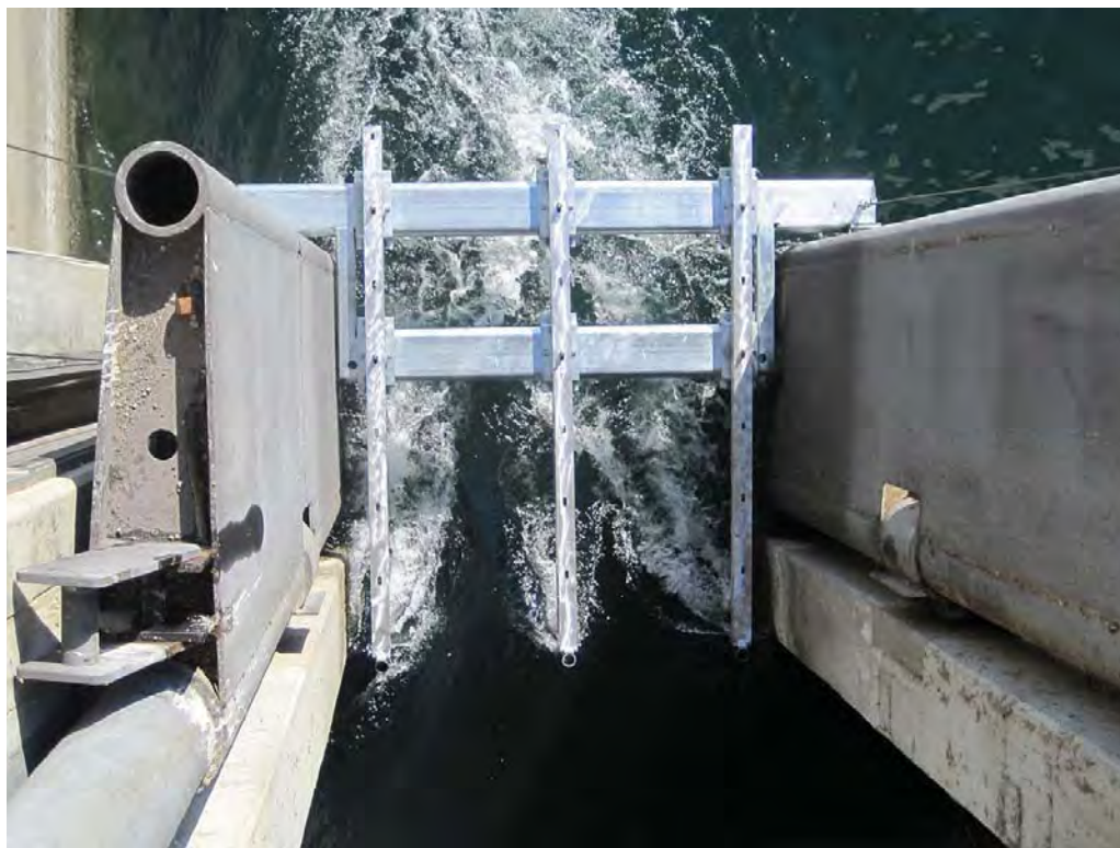
Photo 3: Looking down on the ADV trolley shown inserted in the bulkhead gate slots. (This photo was taken by Jacobs Engineering during the trolley testing in Feb 2011)
