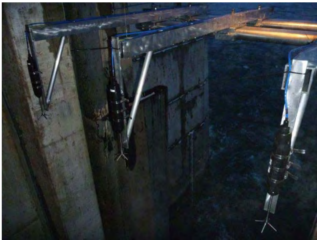
Photo 4: ADVs shown mounted on the support arms prior to being lowered into the water for testing. (Photo by Douglas PUD)
