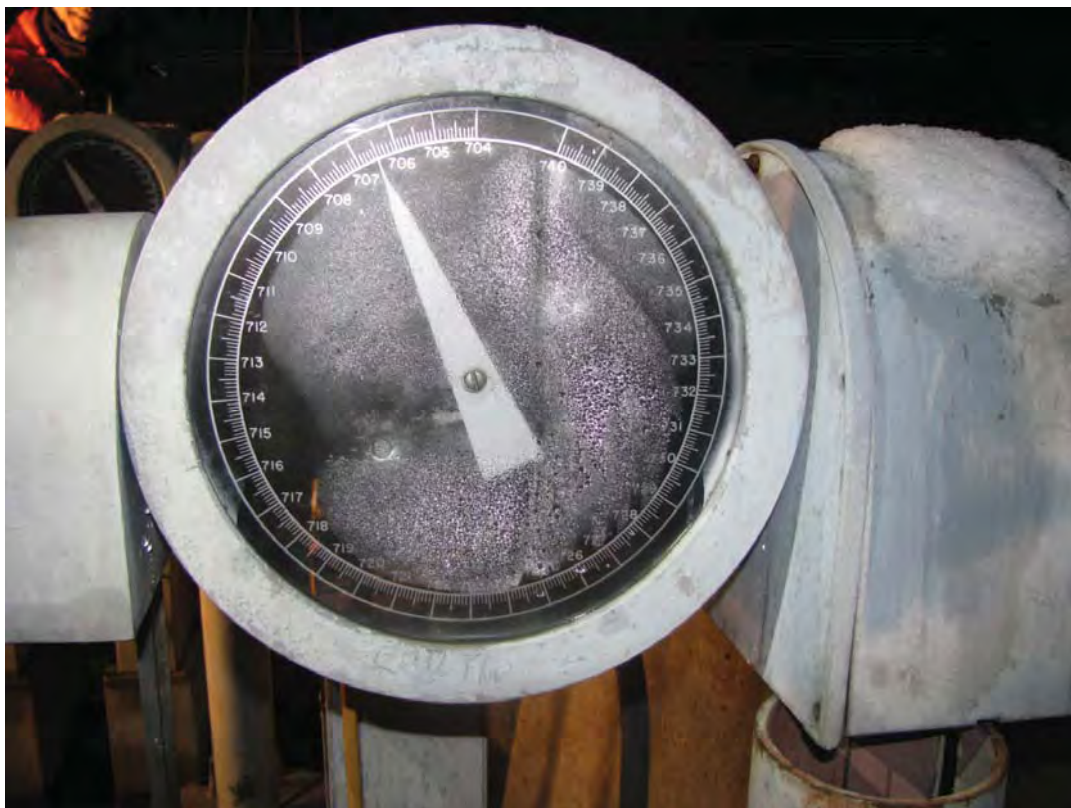
Photo 6: Tailwater gage used to record the tailwater level. The Collection Chamber gage is in the background to the left. The difference between these two readings indicates the head drop across the fishway entrance. (Photo by NHC)
