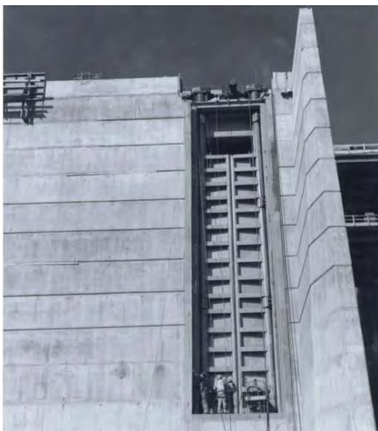
Photo 2: Looking upstream at the de-watered West fishway entrance during maintenance. In this photo the two gates are closed. (Archival Photo from Douglas PUD)
