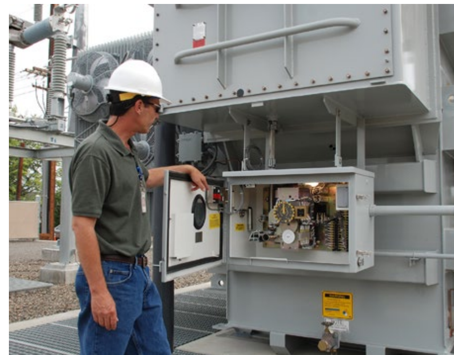
Tom Kelly, senior substation engineer, checks equipment at the new Okanogan Substation in Wenatchee before it was energized in July 2013.
