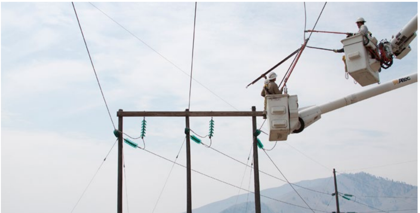
Below: Chelan PUD line crews reconnect transmission lines as part of maintaining high-voltage equipment near Chelan.
