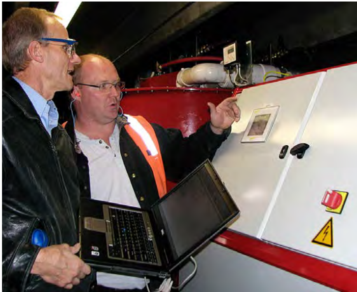
PUD engineer Jim White, left, and James Hursh of Stemilt Growers, check the control panel of a CO 2 scrubber at the fruit company's Wenatchee facility. Energy-saving scrubbers installed with help from the PUD use 95 percent less energy than equipment previously used at the warehouse to keep fruit fresh for long periods of time.
